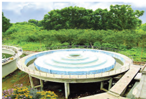
Air mixing tank
